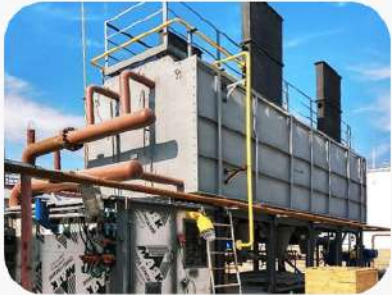
Oil heating furnaces
